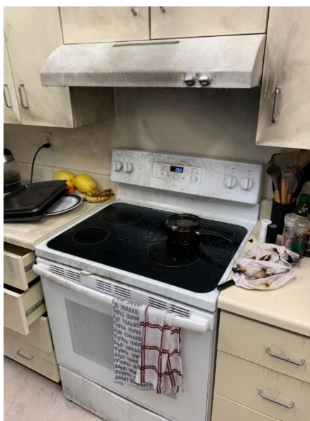
Stove top cooking fire damage
